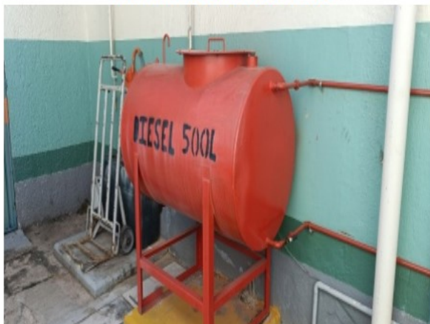
VISTA TANQUE DIESEL
